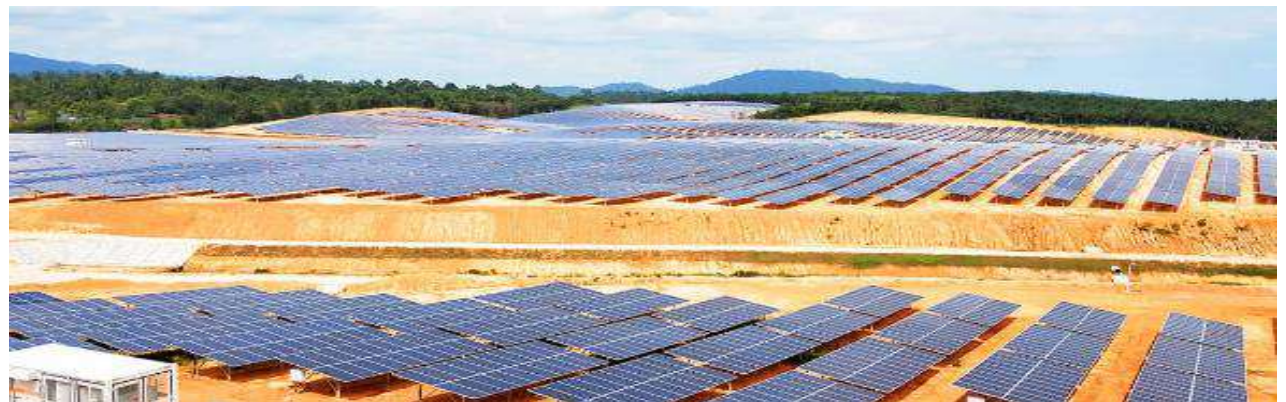
50 MW solar farm at Gambang, Pahang, Malaysia
