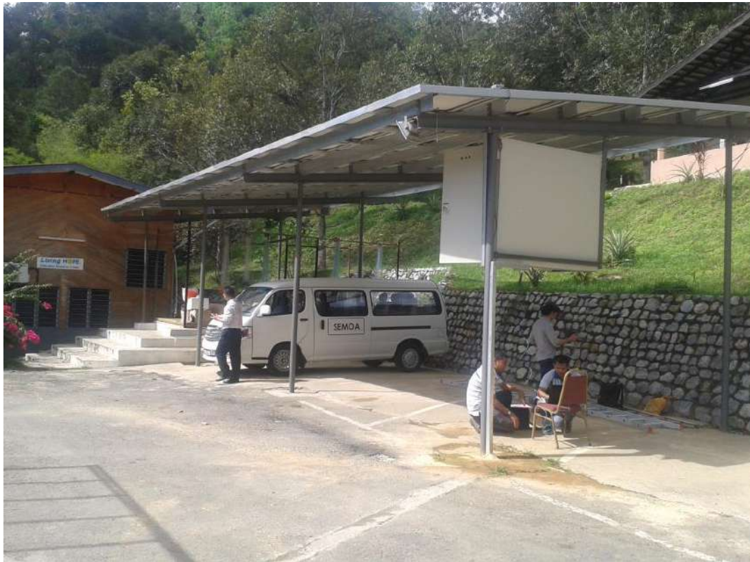
23 kWp grid-connected PV system
