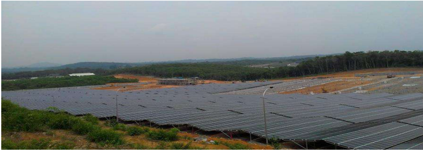
8 MWp solar farm at Melaka, Malaysia
